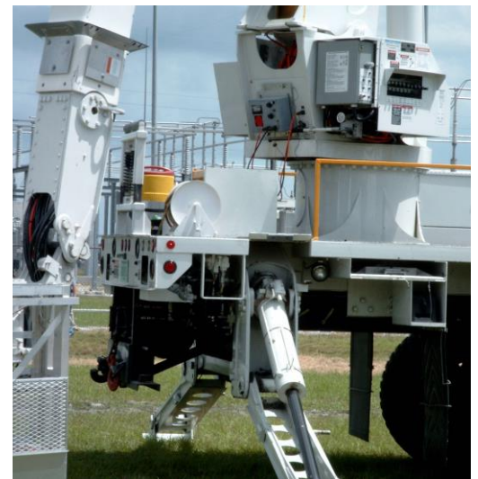
BCM 44B Installed on boom
